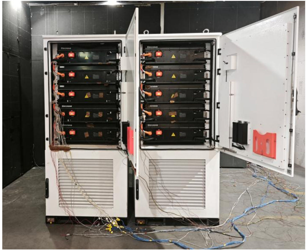
Figure 2 of Attachment 5: overview of units with door opened_after test
