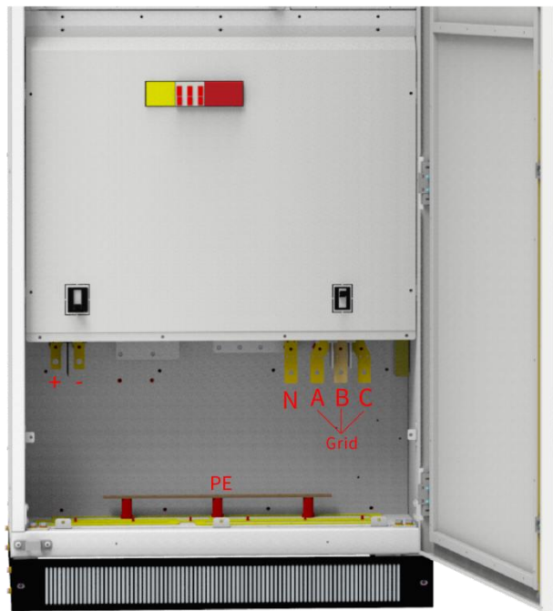
Figure 3-4 Switch block and terminals
